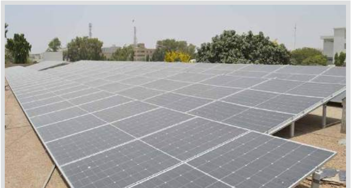
350 kW Solar Power Project (In Progress) – Expanding renewable energy capacity to reduce carbon footprint and grid dependency.
