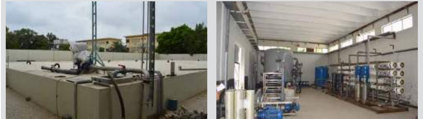
Water Storage Tanks (500,000 IG) – Expanded storage capacity to enhance water security and operational continuity.
