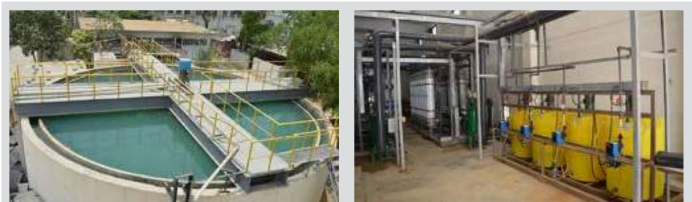
Effluent Treatment Plant (ETP) – Treating industrial wastewater to ensure compliance with stringent environmental discharge standards.
