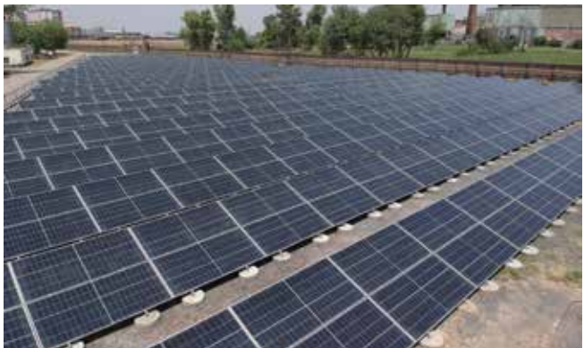
The Polyester Business commissioned a 1 MW solar power system at the Polyester Plant, Sheikhpura.
