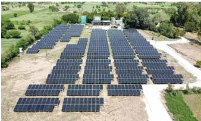
The Soda Ash Business completed Phase 2 of the solar power project at Bela Pumping Station, Khewra through the installation of an additional 250 kW system.
